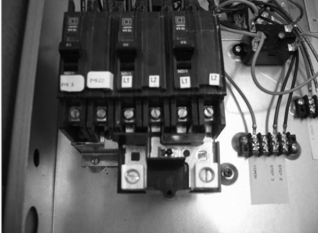
FIGURE 8: JUMPER BAR SHOWN INSTALLED ON CIRCUIT BREAKERS.
